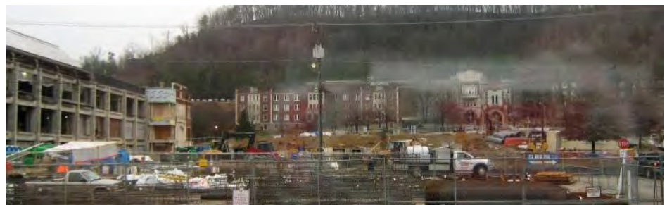
Fields Hall (center) and Camden Carroll Library (right) will be obscured from the church view after ADUC is enlarged.
