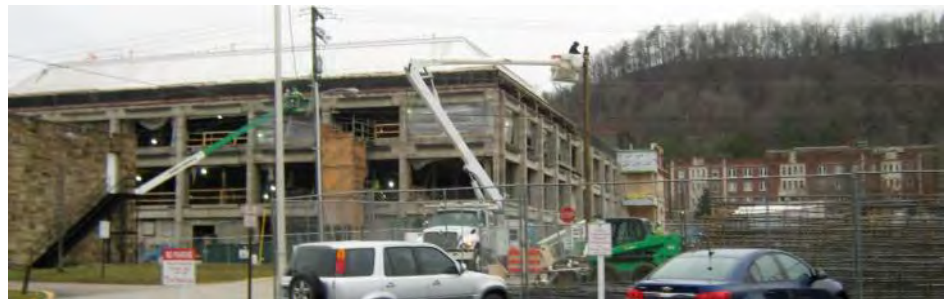
Monarch Construction is in charge of renovation at Adron Doran University Center (ADUC), which will be doubled in size when completed.
